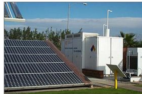
Solar powered electrolysis station in Thousand Palms, CA for fueling fuel cell buses
