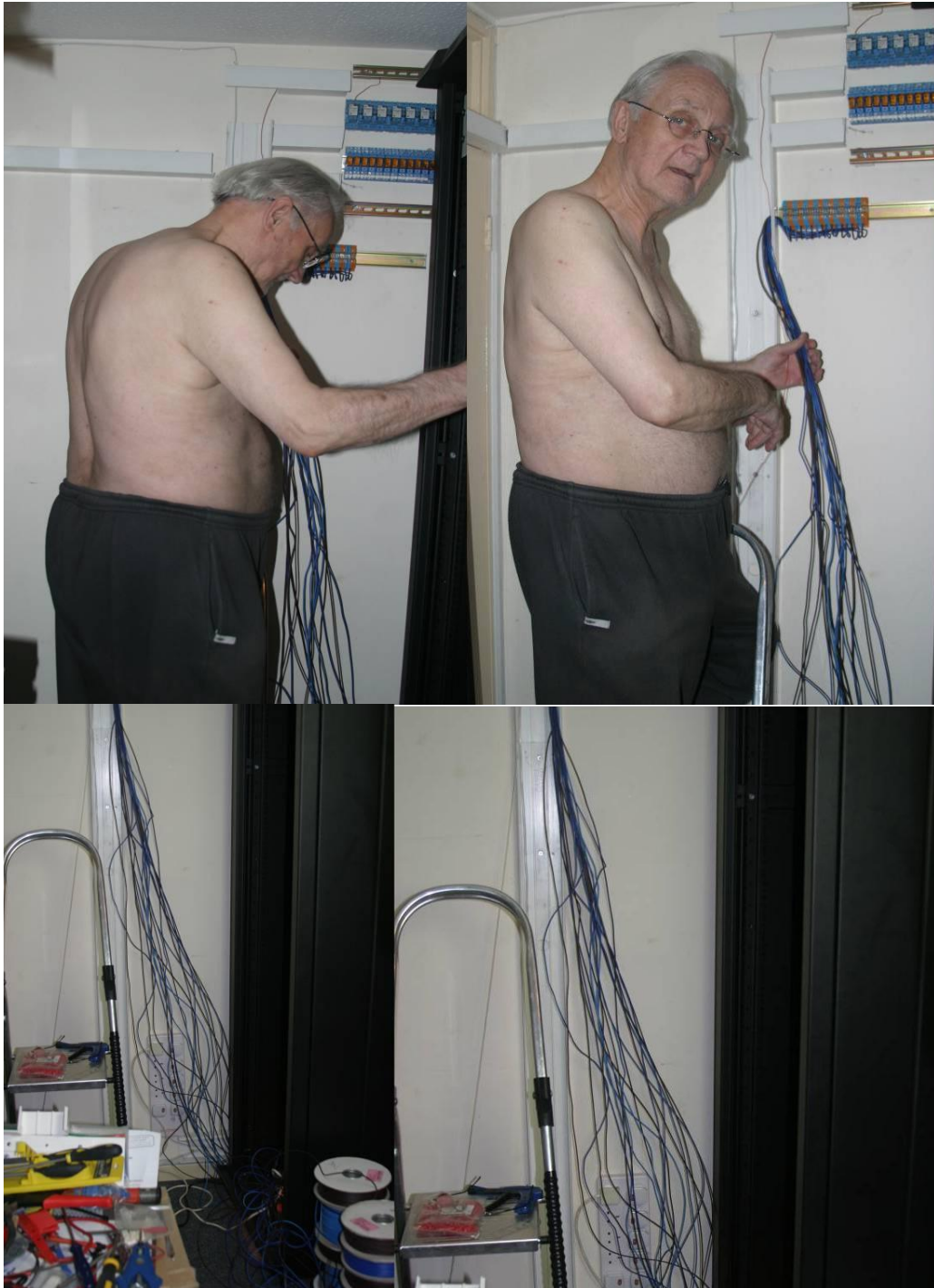
This is cabling without the proper means for such a project.
